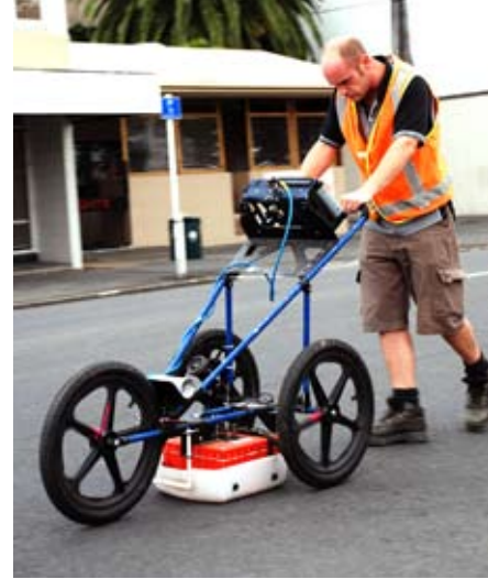
Ground-penetrating radar is used to find underground services
